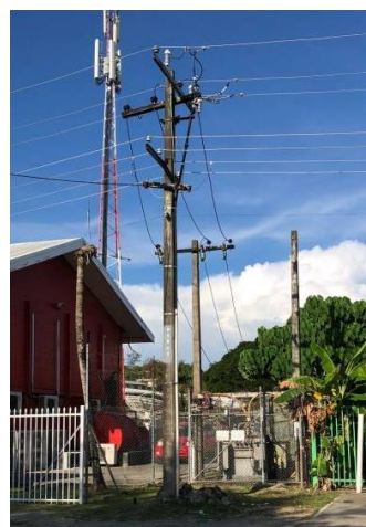
Photo 2-13 Transformer in urban area
