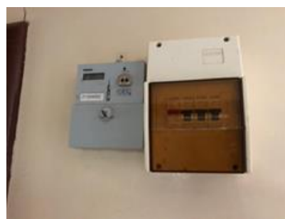
Photo 2-2 Digital kWh Meters
