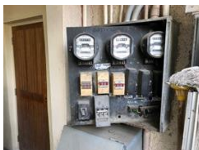
Photo 2-1 Mechanical kWh Meter
