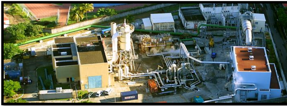
Bouillante Geothermal Power Plant in Guadeloupe (aerial picture, BRGM)
