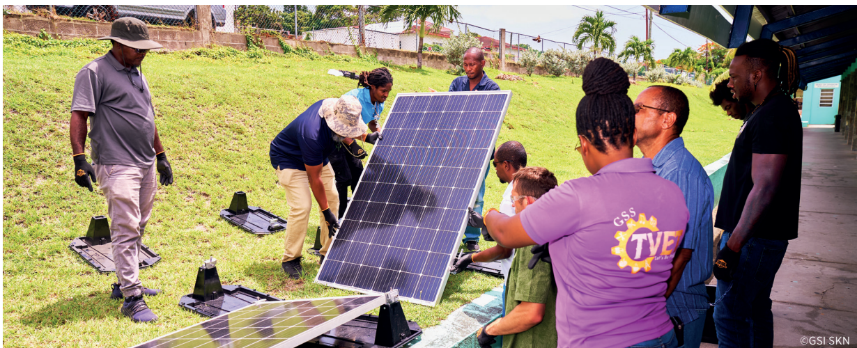
Solar PV technicians being trained in solar PV system operation and maintenance in Saint Kitts and Nevis
